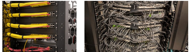
Fig. 1. The operational reality this work targets: densely populated rack switches in production datacenters where up-time targets exceed 99.99%, ports are tightly spaced, and routine cable swaps demand contact-aware manipulation that does not disturb neighboring connectors.
