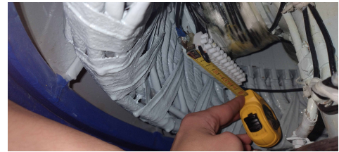
Fig. 7. Auxiliary terminal block with shorting cable used for fault injection via external resistors.
