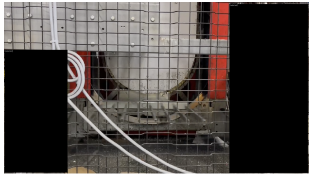
Fig. 7. Facility A lift looking from on the floor
