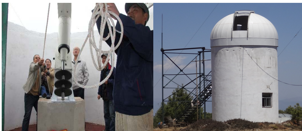
Figure 4. (Left): In the early stages of YOGIS construction in 2013, the coronagraph lacked rainproof facilities. A movable rain shelter was installed on the roof of the circular building. The image shows staff members opening the roof shelter via pulleys to conduct observations. (Right): In 2014, a dome was designed and installed according to the dimensions of the circular building, upgrading the equipment for safeguarding the observation environment.
