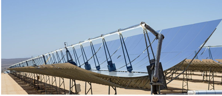
Figure 1: Receiver tubes in a CSP-type solar plant.
