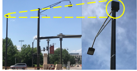
Figure 3: Antenna array placement at the auxiliary site.
