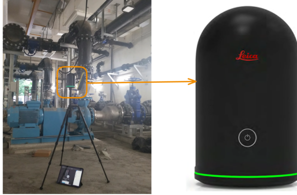
Figure 2: Data acquisition equipment for Industrial3D. The Leica BLK360 terrestrial laser scanner is shown in detail (inset) and deployed in an industrial scene (WRT2), where an iPad Pro controller facilitates real-time preview and registration.
