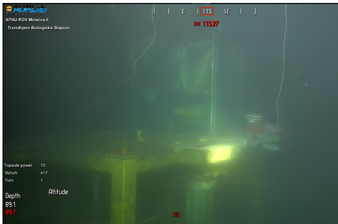
Fig. 14. ROV during manual inspection of the pigloop module on which the docking station is mounted.
