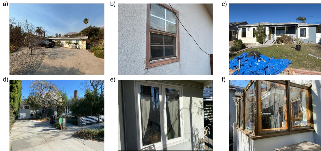
Figure 11: The household in 11 (a – b) and 11 (d – f) were classified as no damage, but the ground truth was affected due to the broken glass. The household in 11 (c) was classified as affected due to the tarp being interpreted by debris; however, the ground truth was no damage.
