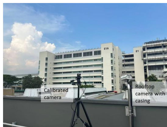
Figure A1: Site photos of calibration on rooftop using a calibrated camera on the left for the installed IR camera on the right.
