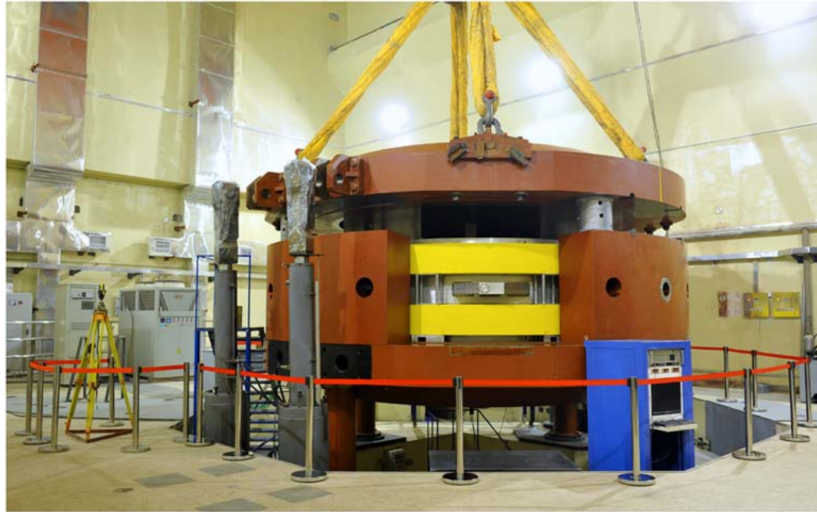
Figure 2.11: Main magnet, main coil, vacuum chamber, and hydraulic elevating equipment after installation.
