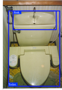
In the image, there is a toilet with its lid up. The toilet is white and has a handle on the side of the toilet itself. There is also a small amount of water coming out of it. The image also shows a pipe running along the wall. It is located in the bottom left corner. Overall, this image captures a moment in a bathroom setting.
