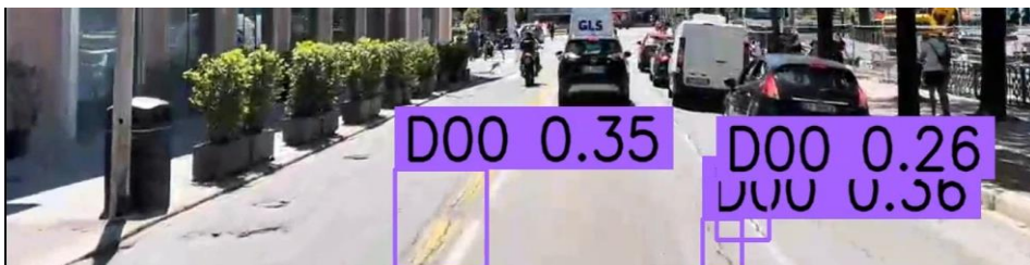
Fig. 2. Road damage detection
