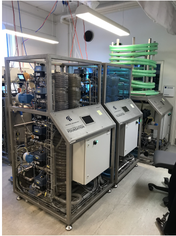
(a) On the left are two pipe units. These units measure volume flow rates and pressures, and can be configured for pipe sections of varying lengths. On the right is a pumping station, where water is pumped from a water reservoir into the system, until finally returning to the reservoir.
