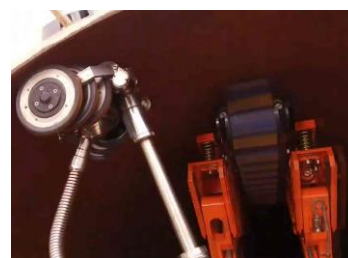
Figure 15. Zoom on a probe and the top crawler deployed against the pipe inner surface
