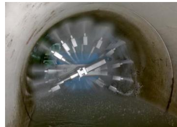
Figure 9. SVM-RS cleaning tool at rear [14]
