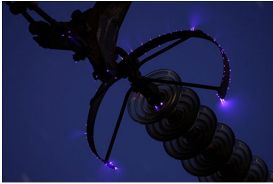
Fig. 1. Corona discharge on corona ring of 500 kV overhead power line
