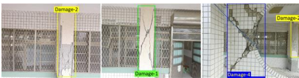
(b) damage level classification for earthquake reconnaissance (Damage 1 – surface crack, Damage 2 – spalling, Damage 3 – spalling with exposed rebars, and Damage 4 – severely buckled rebars) (adapted from [58])
