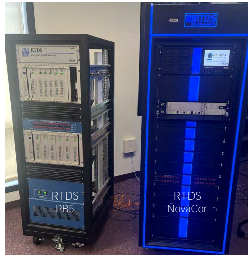
Fig. 1. NovaCor and PB5 racks of the RTDS setup.
