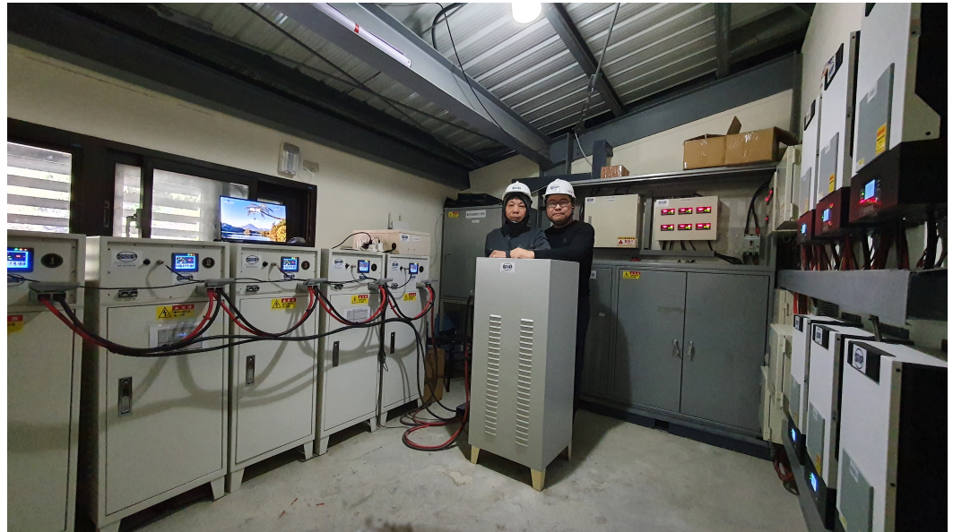
Figure 11. Site photo after the completion of the off-grid PV ESS improvement (The photo was taken on Oct. 10th, 2022). The ESS consisting of 6 energy storage cabinets is on the left side, and the hybrid solar inverters with major distribution boxes are on the right side. The people standing in the middle are Jung-Feng Jack Lin (left) and Hsien-Ching Chung (right).
