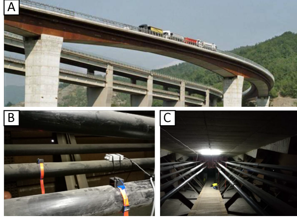
Figure 2: A) Aerial view of the viaduct under analysis. B) Sensor positioning on prestressing cables. C) Prestressing cables.
