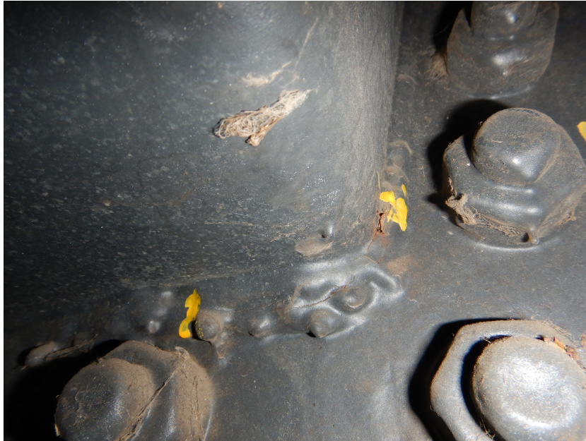
Fig. 1: Example of a steel bridge structure image where common crack detection algorithms tend to have a high false call rate.
