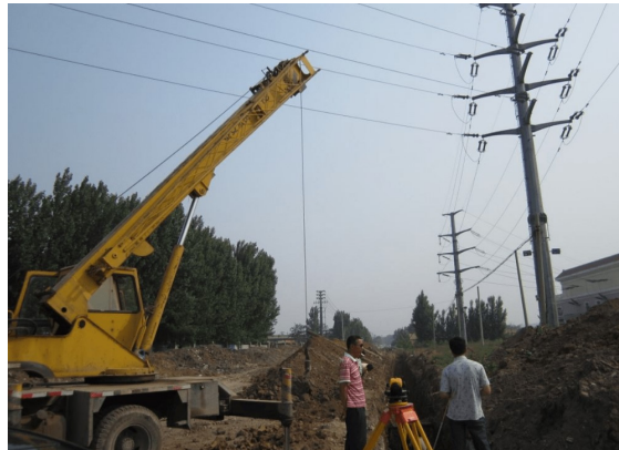
Figure S11: Electrical project site. Taken from 7 .
