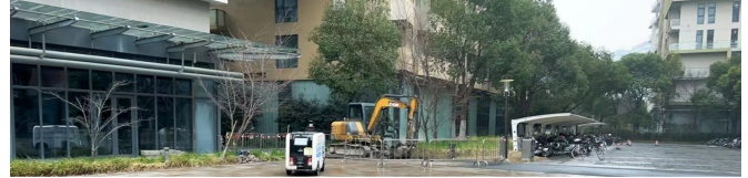
Notice about Emergency Repair of Sewage Pipes on the East Side of the Silk Road Canteen and Road Closures
