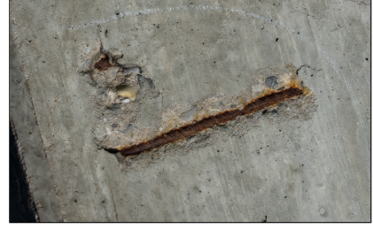
(a) Textured mesh showing an exposed reinforcement bar.
