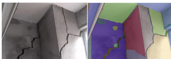
Figure 1 Example image of directly applying SAM for crack segmentation.
