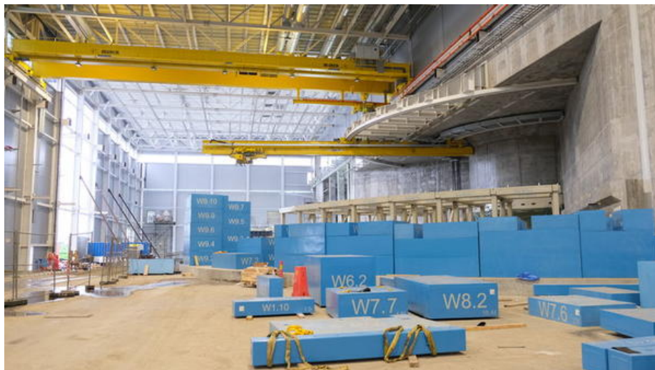
Figure 5: Overview of the complete bunker area in the ESS D03 instrument hall.
