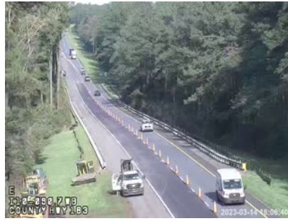
(e) Road construction with a closed lane, affecting traffic routing and conditions
