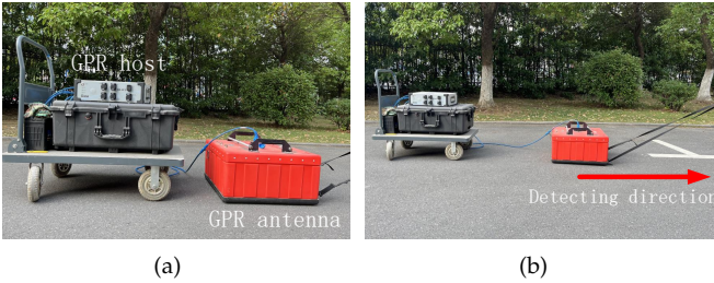
Fig. 9. (a) shows the host and antenna of the utilized GPR. (b) shows the actual detection scene of a road. The GPR antenna is moved along the road (the red arrow) to obtain the GPR B-scan image, and the collected image is transformed to the host. As mentioned in the background, each column on the B-scan represents a received electromagnetic wave, and there is a sequence and connection between the columns in detection time or position.
