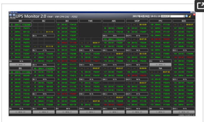
Figure 16. UPS (Uninterruptible Power Supply) monitoring system.
