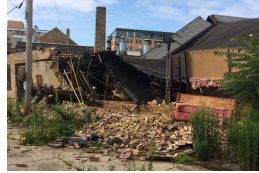
(c) Ridge Avenue is closed after a partial building collapse and electrical fire Saturday night. (negative)
