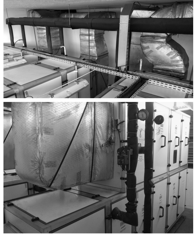
Figure 2: Photos of the AHU room depicting the air ducts (top), the supply and return water pipes (top and bottom), and the three-way valve servomotor (bottom).
