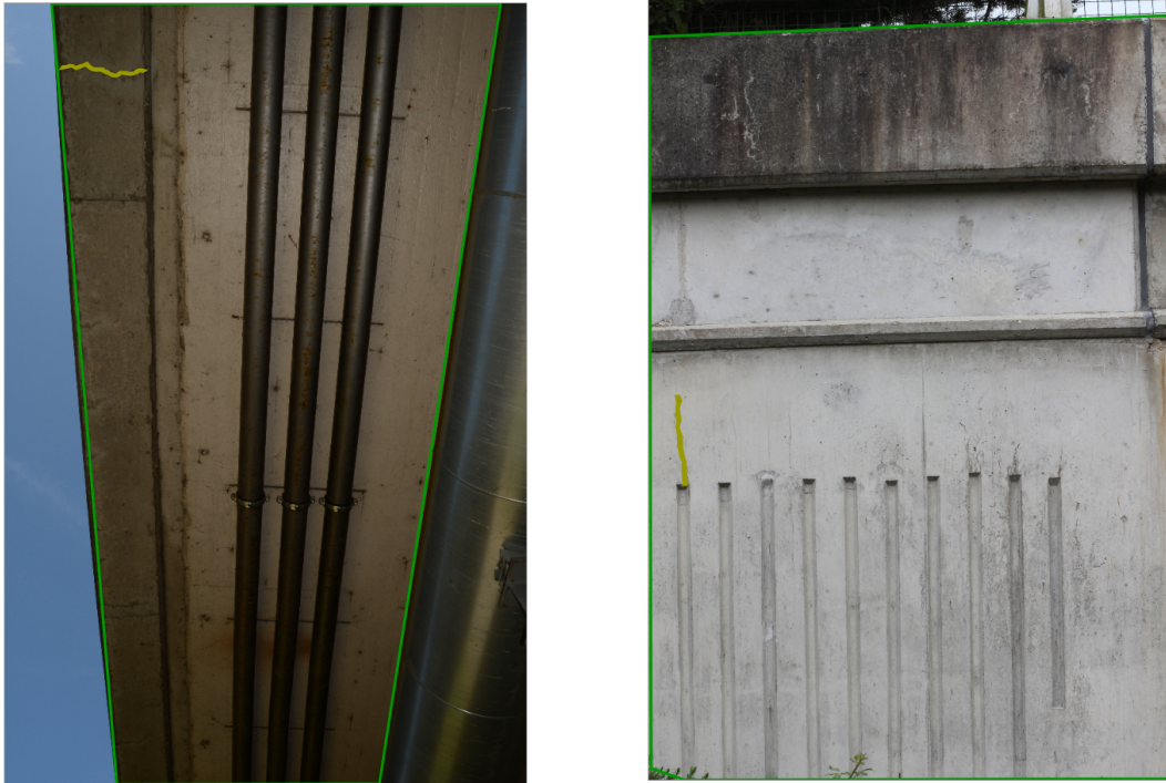
Fig. 1: Example Crack Regions in Infrastructures, annotated with Yellow-colored pixels
