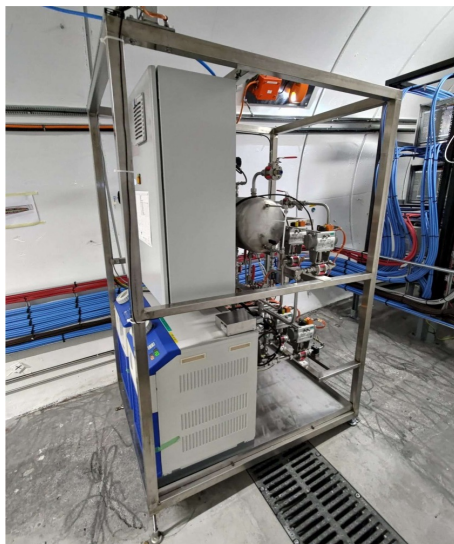
Figure 13: Photograph of the cooling system.
