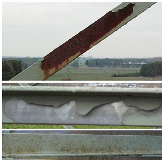
Figure 1: Examples of a corrosion damage, a missing painting damage and a patch of dirt, from top to bottom.
