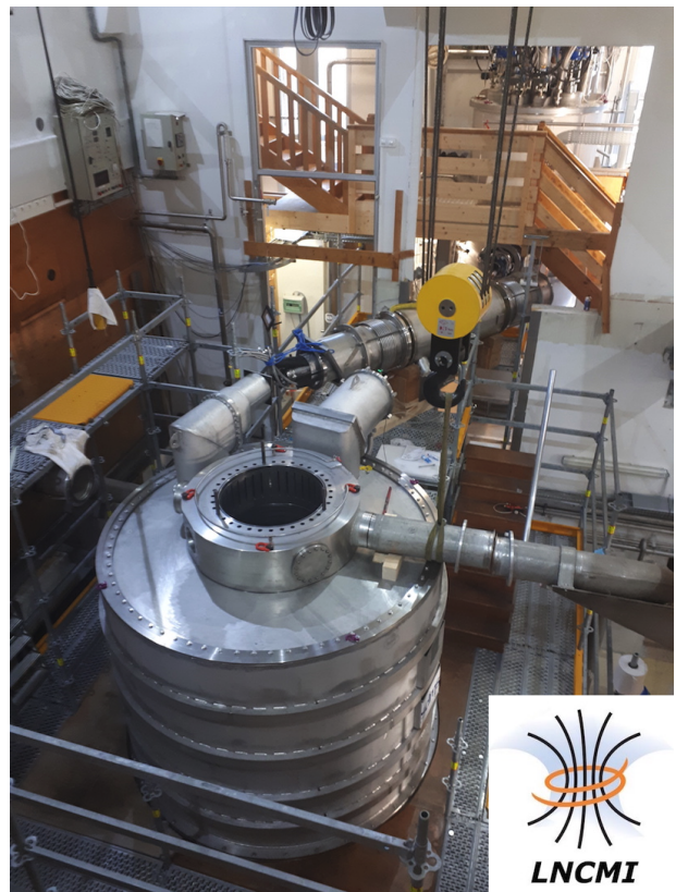
FIG. 1. Status of the construction of the Grenoble hybrid magnet. In the front : assembled magnet cryostat with its warm bore diameter of 812 mm. It contains the superconducting coil immersed inside its 1.8 K He vessel and surrounded by three thermal shields at 4 K, 30 K and 100 K. On the top of the magnet cryostat, one of the water cooling pipe for resistive magnets is being connected. In the back : the cryogenic line to be connected to the magnet cryostat and to the cryogenic satellite producing the superfluid He can also be seen. Final assembly : beginning of 2022. First operation : beginning of 2023.
