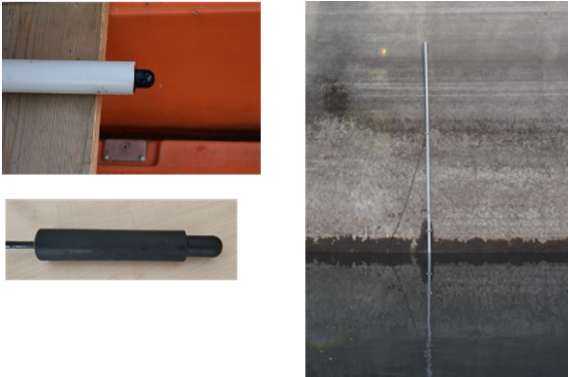
Fig. 1. Upper Left: Hydrophone inserted in a plastic pipe. Lower Left: The hydrophone. Right: The installation of the hydrophone on the barrage.
