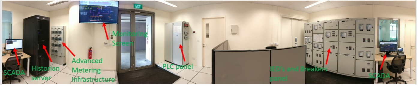
Figure 3: EPIC control room, 360-degree view. The picture shows different physical components including the SCADA workstation, IED and Breaker panel, PLC panel, Historian server, Advanced Metering Infrastructure (AMI) and the Monitoring screen.
