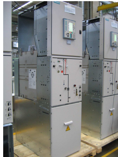
Fig. 1. A typical electric switchboard (Wikimedia, https://commons.wikimedia.org/wiki/File:Medium_voltage_panel.jpg ; Retrieved 05/01/2021)
