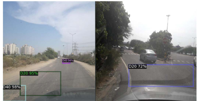
Fig. 13. (left) Damage detection far away on the road surface may not represent the actual damage and raise false positives. (right) Image has dashboard reflection artifacts which is falsely classified as a damage.
