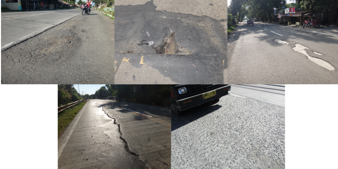
Figure 2. DPWH dataset: Alligator, Bowl-shaped depression, Delamination, Crack, Scaling (from left to right)
