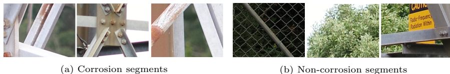
Figure 5: Example of Corrosion and non-corrosion segments
