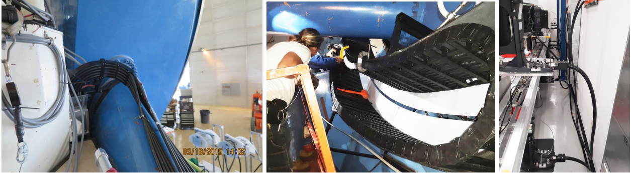
Figure 6. Routing of the cables through the Dec and Polar Axis before they penetrate the wall of the spectrograph shack.
