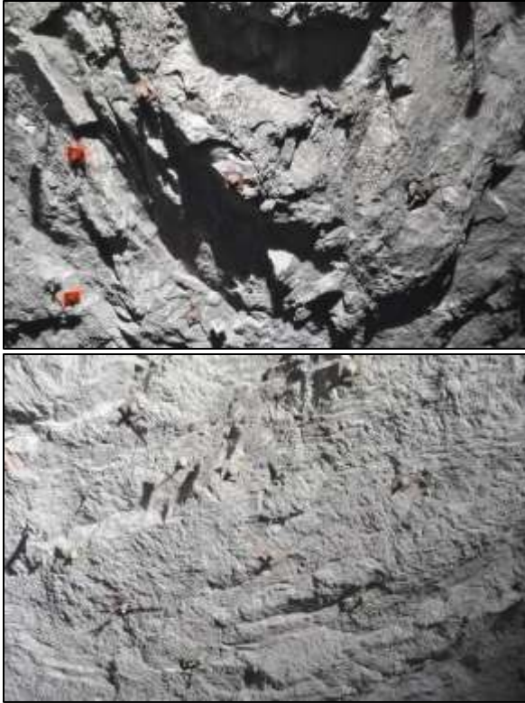
Figure 9. Example images; Hazardous roof (left), Non-hazardous roof (right).
