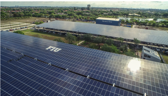
Fig. 7: 1.4 MW PV Located on FIU Engineering Campus used for data collection
