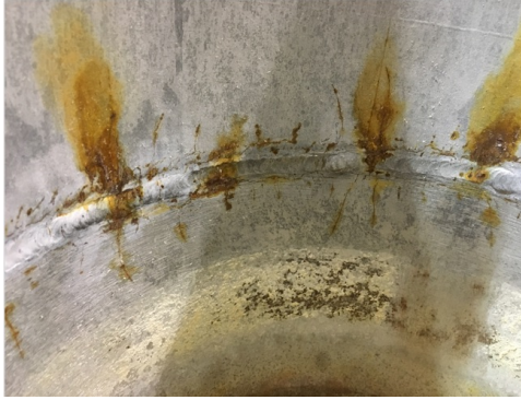
Figure 2: Example image with visible corrosion, stress corrosion cracks, and artifacts (scratches, shadows, etc.). Note: this is a laboratory corroded stainless steel sample and not an image from an actual used fuel canister; to the best of our knowledge no canisters have been detected with defects).
