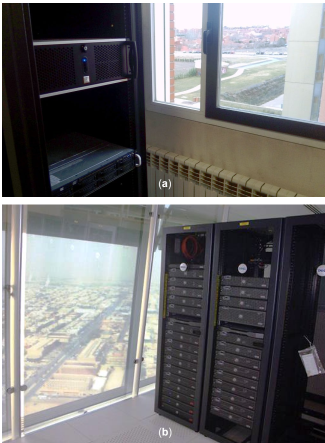
FIG. 1. Server racks with a view to the outside. (a) A picture taken at author's (J.C.G.-E.'s) own university. (b) Computer server room in Al-Faisilya Tower, Riyadh, Saudi Arabia [37].
