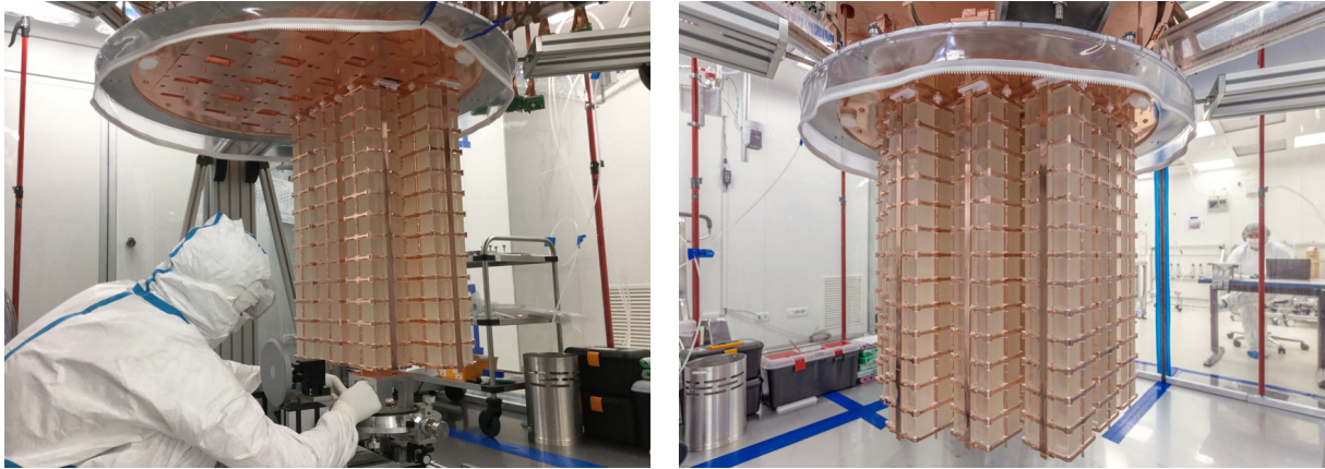
Figure 19: Installation of the CUORE towers. The top part of the plastic radon bag is visible around the tower support plate. Left: an operator positions a tower using the cart. Right: tower installation completed.
