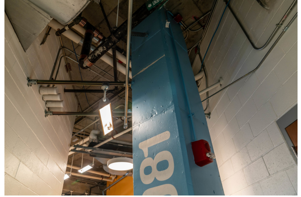
(b) Photograph of the pipes and ventilation system in the basement.
