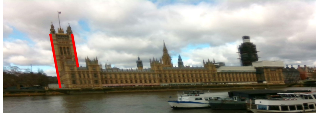
(a) The tower leans towards the left direction.
