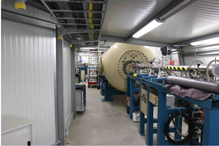
Fig. 8. View of the accelerator room underground, including the high voltage tank of the 5 MV Pelletron. The beam lines are already placed in the tunnel, but not yet aligned and connected.
